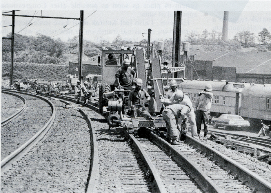
Track work began at 11 locations in six states on April 2 as the Northeast Corridor Improvement Project began its third construction season.
